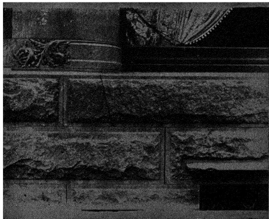
FIG. 197. — Sandstone broken by transverse strain, caused by settling of the building.
