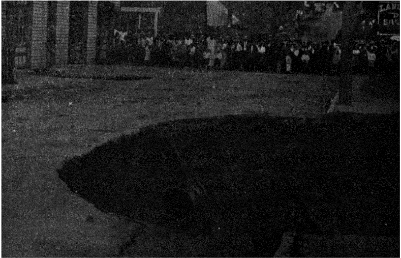
PLATE XLVII, FIG. 1. — Street in Staunton, Va., showing sewer pipe whose break started the caving, and holes formed in pavement.
