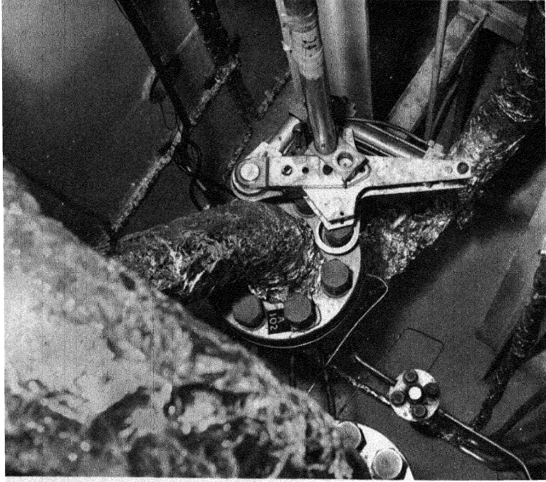
FIG. 7-22. Hydraulic torque wrench for loosening or tightening flange bolts. Shown in operation on HRE-2.
