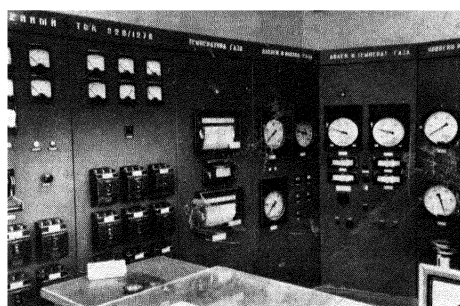
Figure 28. Panel of loop with air cooling
