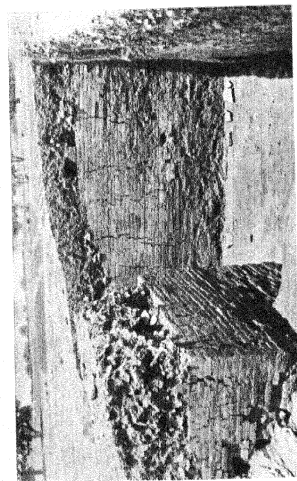
(6) Monastery No. 11: Holes for Beams in the Wall of the S.W. Corner of Verandah.
