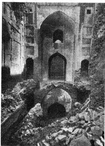
(e) Khariar: Akbar's Tomb from N.E. showing collapsed Frontage.
