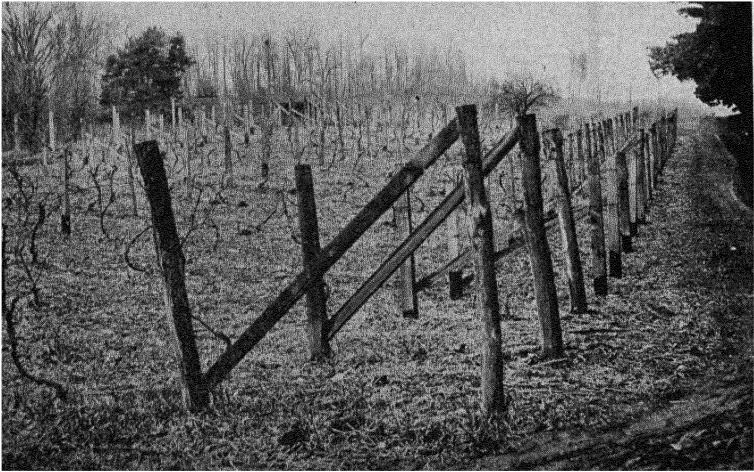
FIG. 188.—A poor type of bracing. These braces are too short and are placed so as to make too acute an angle with the end posts. Such bracing is sure to lift the posts.
