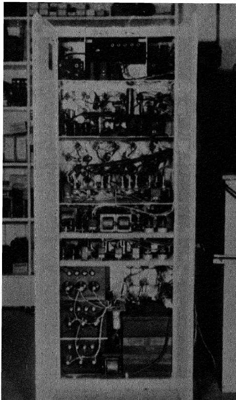
Fig. 7—Back view of the cabinet containing the current and voltage regulators.
