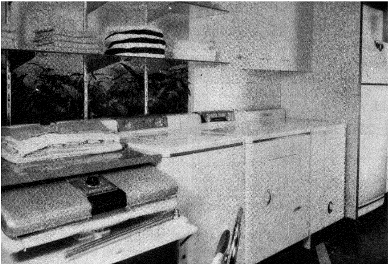
Fig. 8.17. Plumbing fixtures for the laundry include the automatic washer and hot water tank. Note also the dryer and ironer. (Courtesy General Electric Company)
