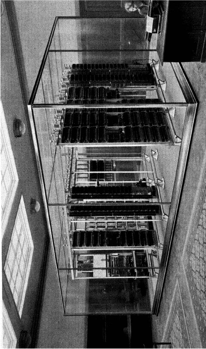
Automatic house exchange in a large German work.
