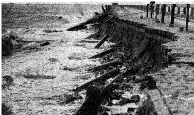
FIG. 5. Destruction of the Nordstrand Dyke after successive tidal surges on October 27, 1936. (Photograph: A. Busch, Morsumhafen.)
