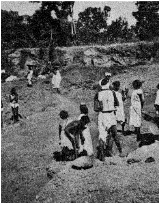
Fig. 2— Showing the Champi bauxite quarry, Bagru Plateau near Lohardaga, Ranchi District, Bihar. (Photo: Vishwa Nath Chhibber).
